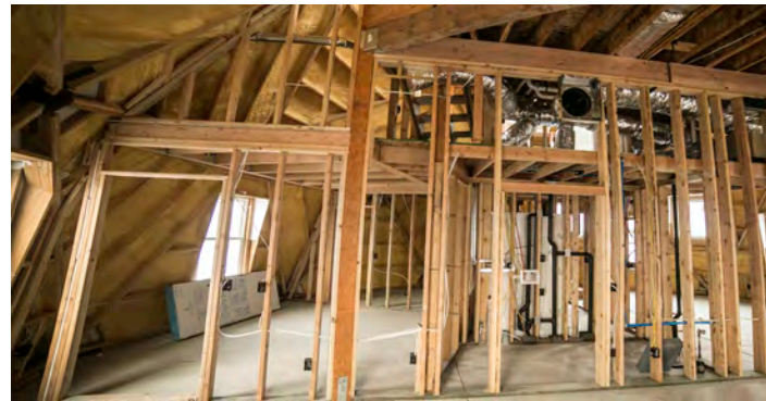
By locating the mechanical room in the Haven's center, the length of the plumbing and HVAC runs are short. The return air is set high in the living room, allowing for the circulation of warm air from the pellet stove.
