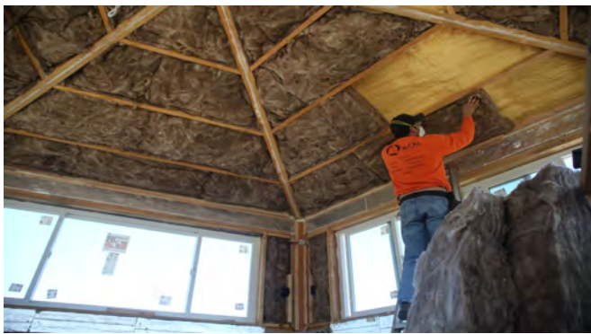
A combination of closed cell foam and fiberglass insulation, provide a high R value thermal break.
